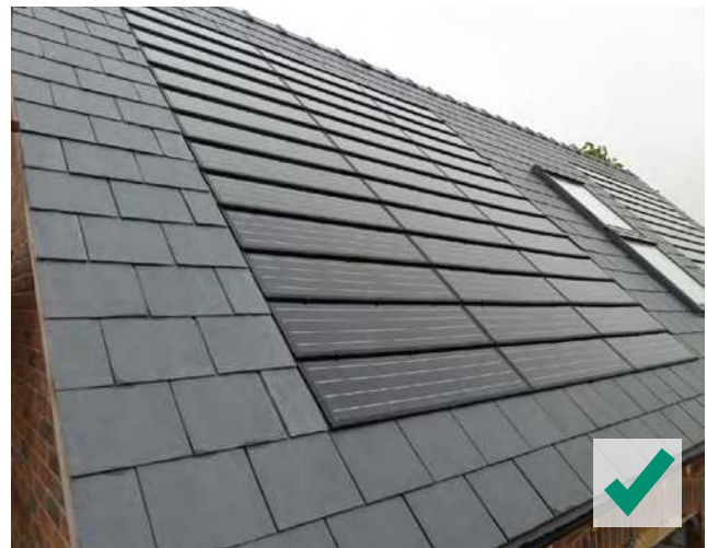
Figure 47: Integrated solar panels on slate roof.
